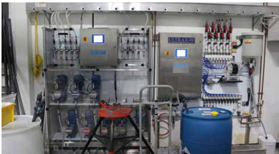
ABOVE: (from top) an employee unloads clean, wet goods from a washer/extractor; a view of three dryers and an automated shuttle that the company has fenced off for safety purposes; a view of the plant's chemical injection equipment.
